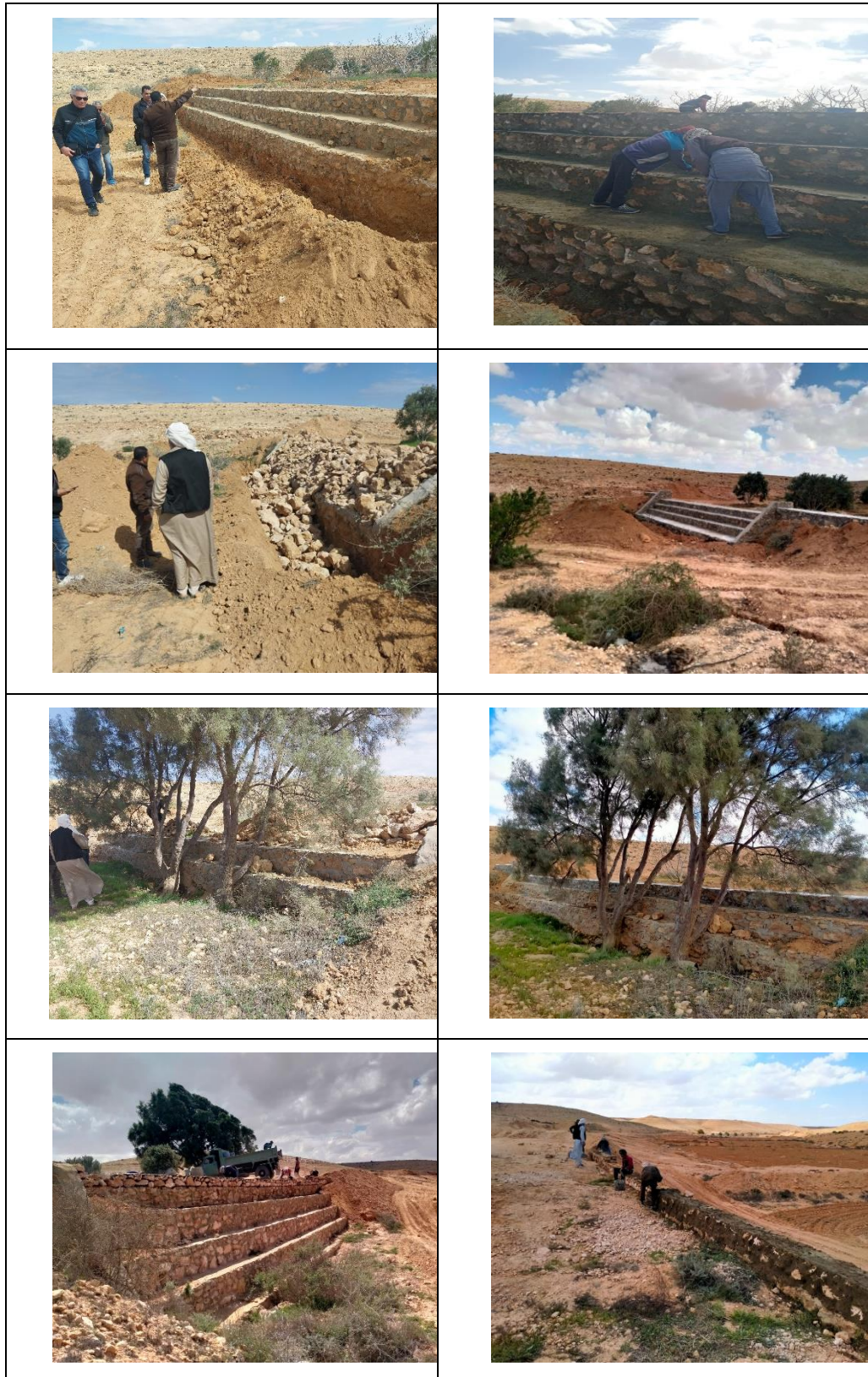
Figure 29. Field Photos for the processes of building and rehabilitation of the dikes
