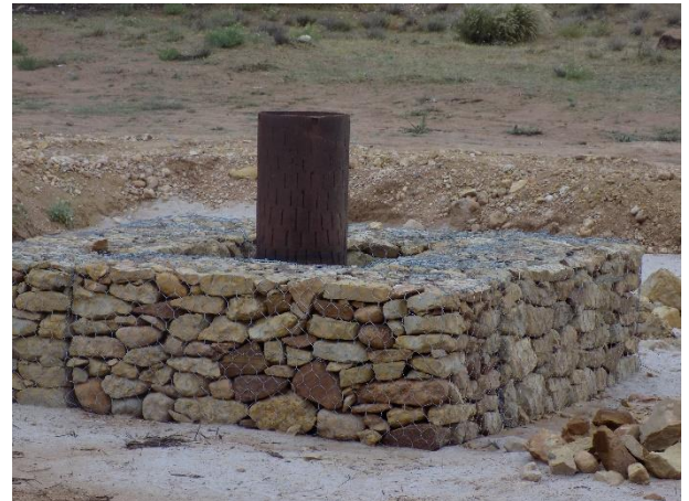
Figure 12. Realization of recharge chamber
